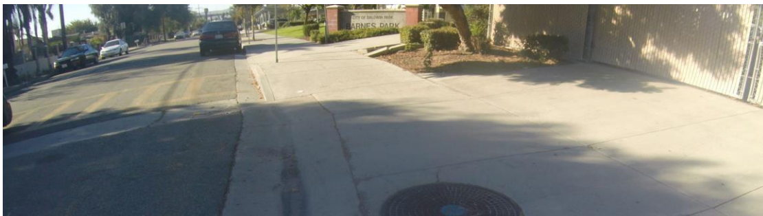
Figure 1-2. Manhole along exist. storm drain running west on Bess Ave, adjacent to the north side of the park
